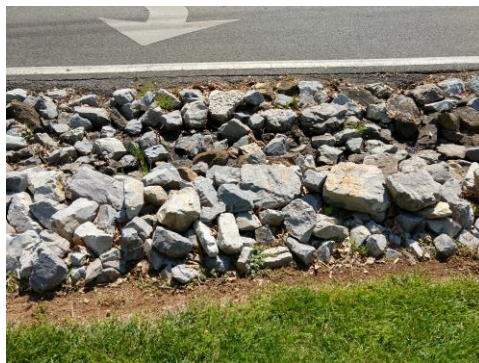
Stone ditch with erosion
