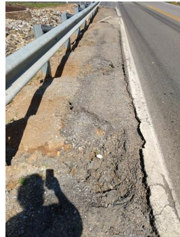
Erosion around guard rail
