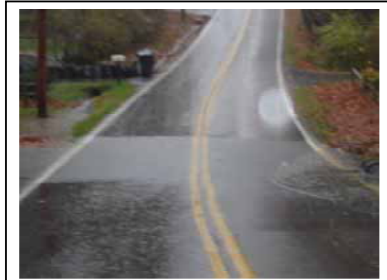
Figure 4. Flooded roadway caused by leaves blocking the storm drainage ditch.
