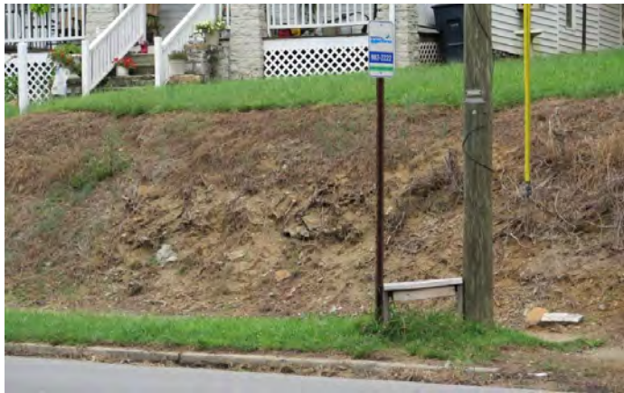
Figure 7.1-2 | Makeshift pedestrian facilities at bus stops
