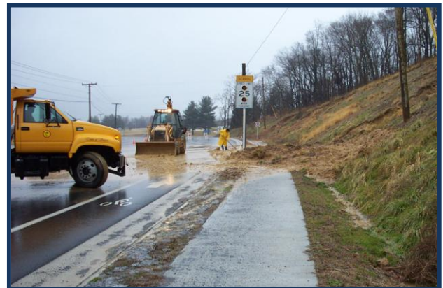
Image 4.13 The Town of Vinton cleans up a mudslide on Hardy Road following a flood in 2003.
