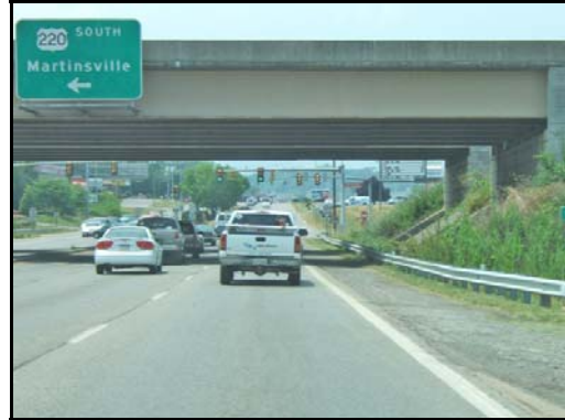
U.S. Route 220 bridge over of Electric Road is a travelway for pedestrians and bicyclists.
