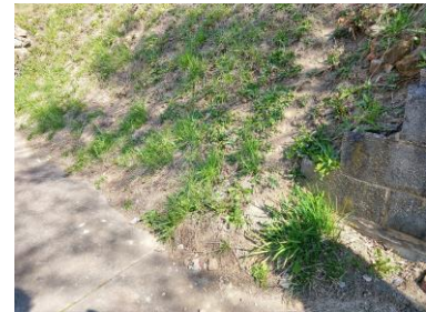
Collapsed retaining wall
