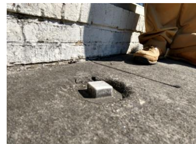
Protrusions like this are a trip hazard
