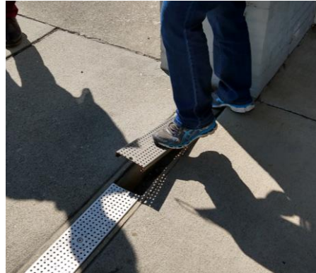
Loose drain cover
