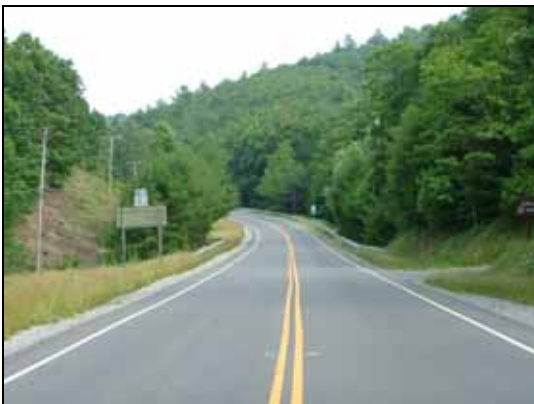
Figure 5.4: Paved should on Route 311 in Craig County.
