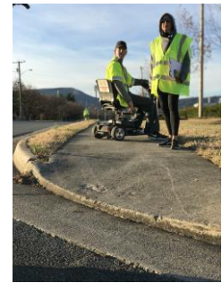
Curb ramp is offset > 1 inch, difficult for wheels
