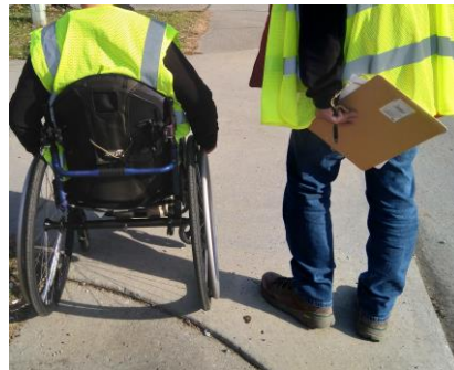
Steep cross slope at drive
