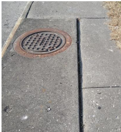
Uneven pavement at storm drain
