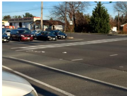
High visibility crosswalk on one leg of Hersherberger and a regular crosswalk on the other
