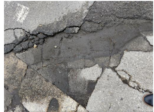
Figure 2. Uneven surfaces challenge people with disabilities and are common at the interface of curb ramps and street
