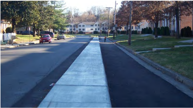
Figure 22: Adding no new impervious surfaces, Westside Boulevard was redesigned to accommodate pedestrians/bikes within the existing street pavement along a path separated from traffic by a concrete median, City of Roanoke
